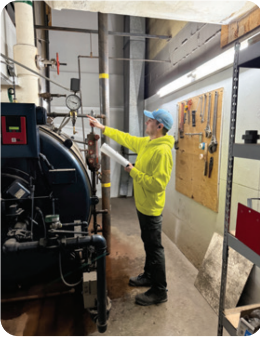
Maintenance check at the WDM Curatorial and Corporate Services Centre
